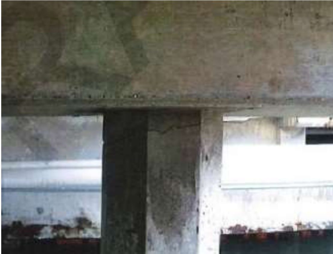
Prestressed Concrete Pile with Horizontal Structural Crack
