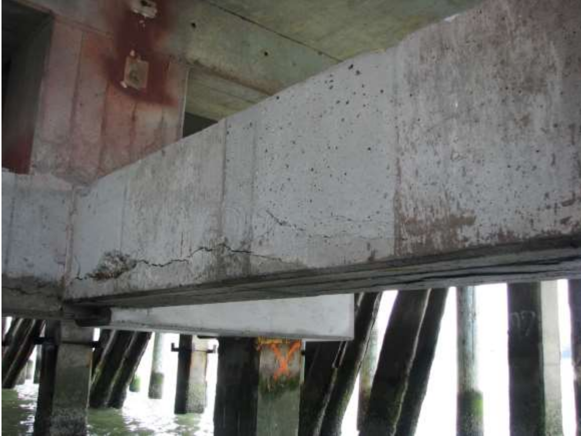
Concrete Beam with Cracks & Open Spall
