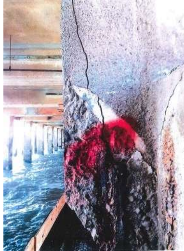
Concrete Column with Open/Closed Spall & Corroded Rebar
