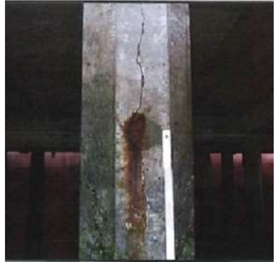
Prestressed Concrete Pile with Vertical Crack & Rust Stains
