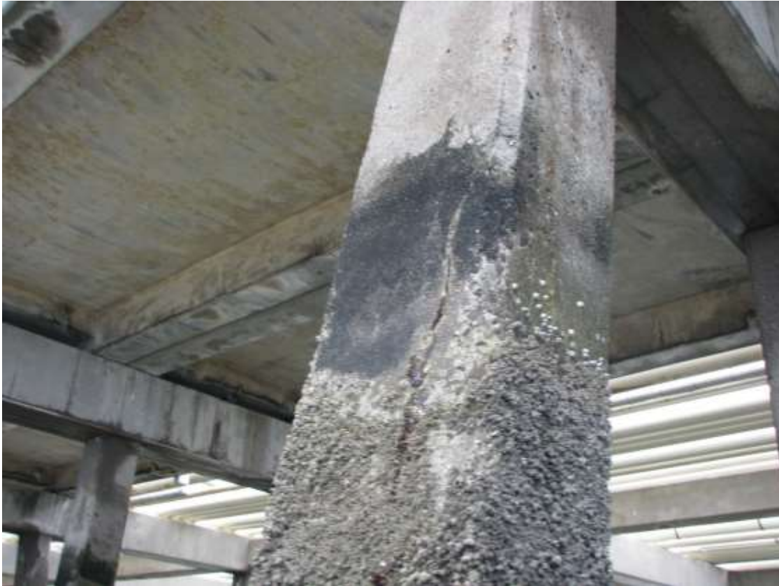
Reinforced Concrete Pile with Vertical Crack
