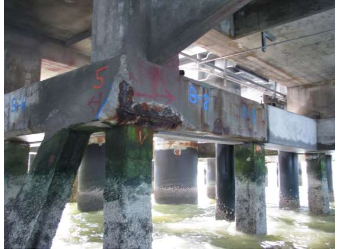
Concrete Beam with Corner Open Spall & Exposed Corroded Rebar
