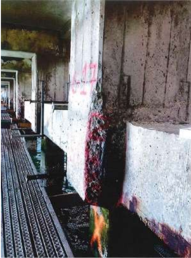
Concrete Column with Open Spall & Corroded Rebar
