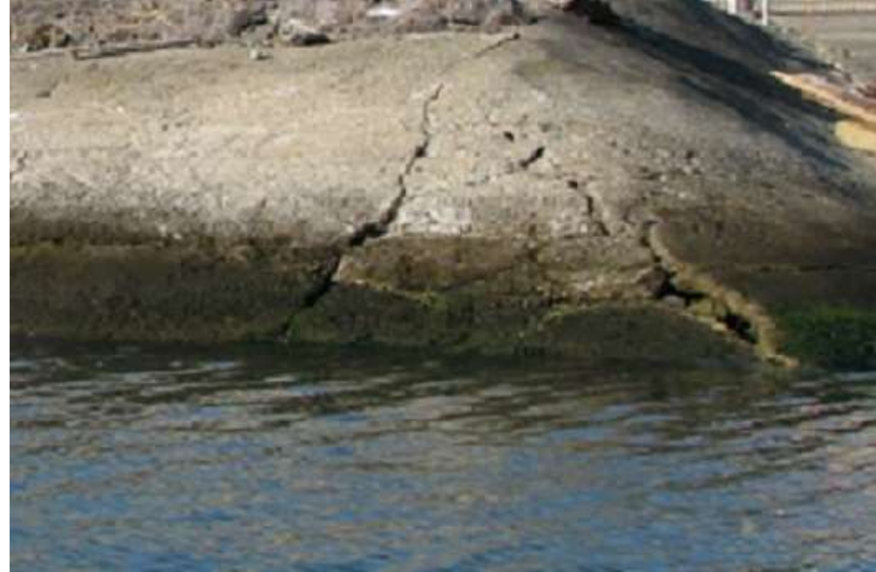
Slope Protection Cracks
