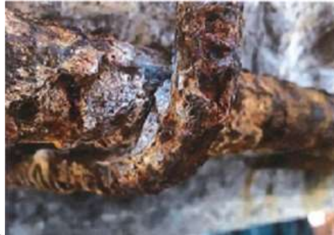
Beam Corroded Rebars
