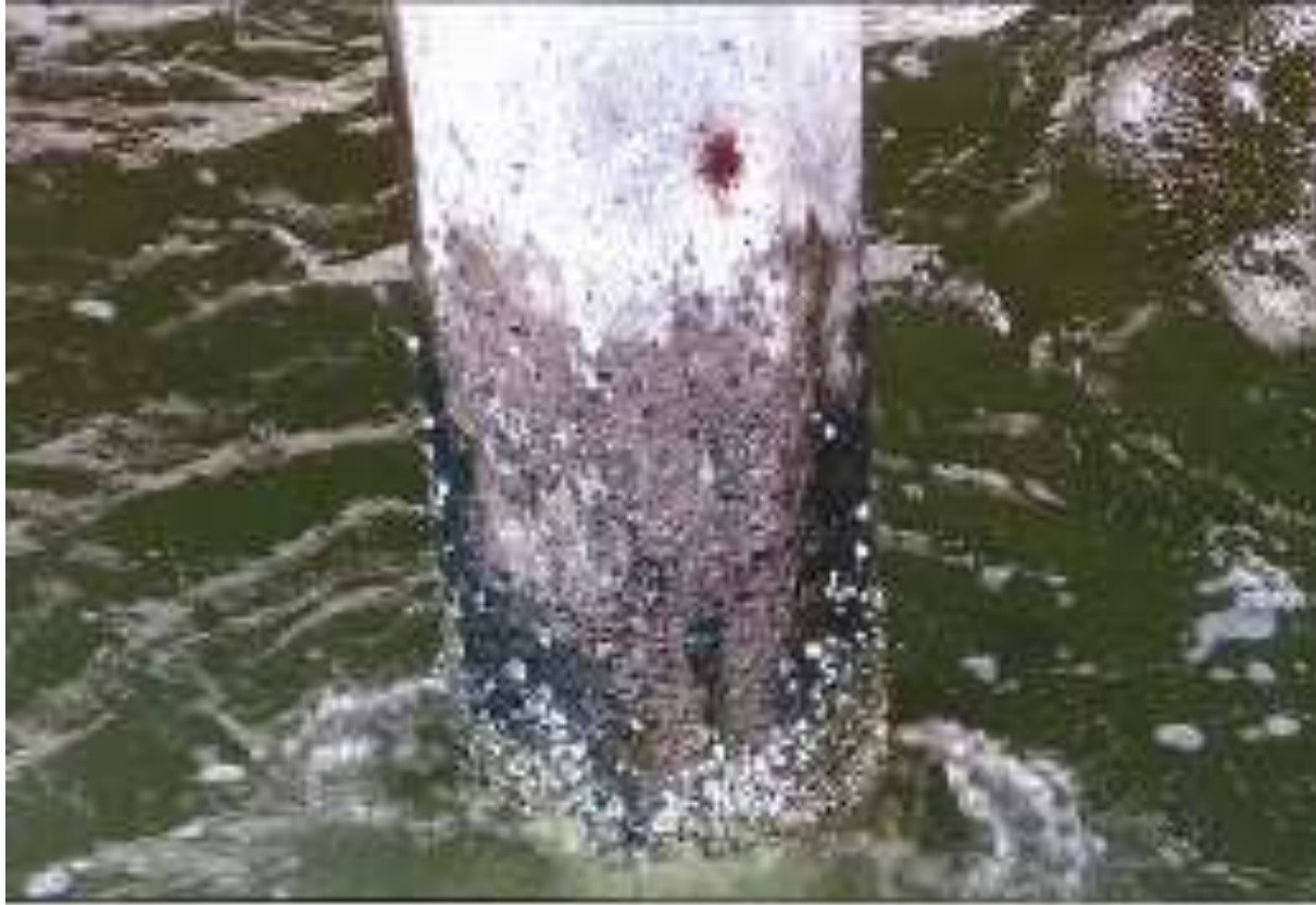
Prestressed Concrete Pile with Pitting
