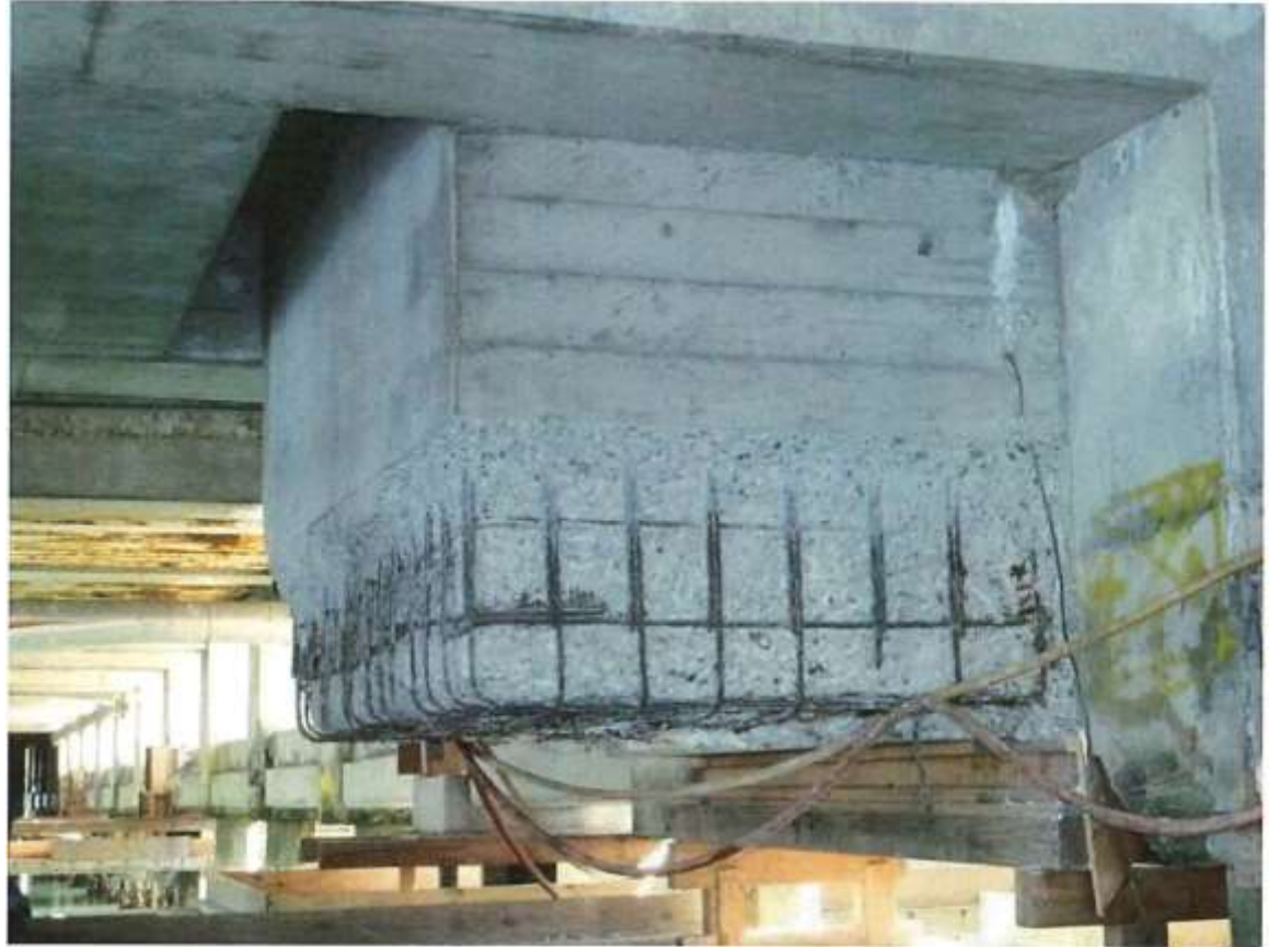
Utility Vault with Soffit & Wall Damage Being Repaired
