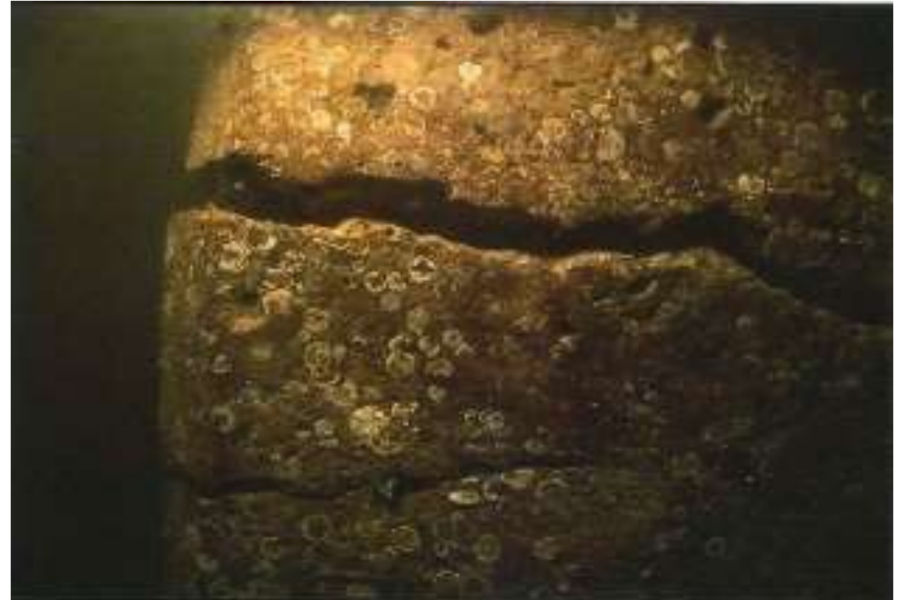
Reinforced Concrete Pile with Breakage from Object Impact
