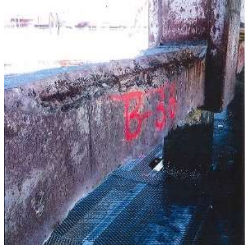
Concrete Beam with Open Spall & Exposed Corroded Rebar
