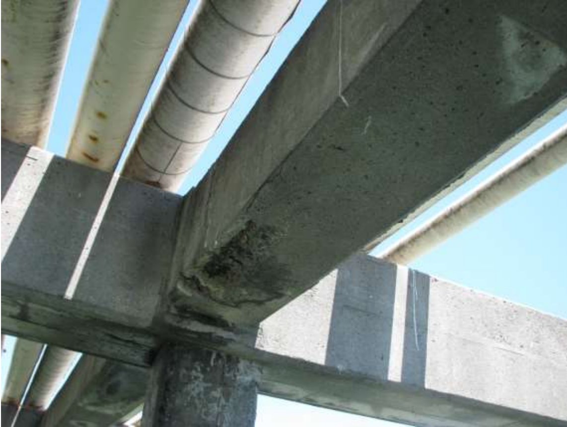
Concrete Beam with Open Soffit Spall & Exposed Corroded Rebar
