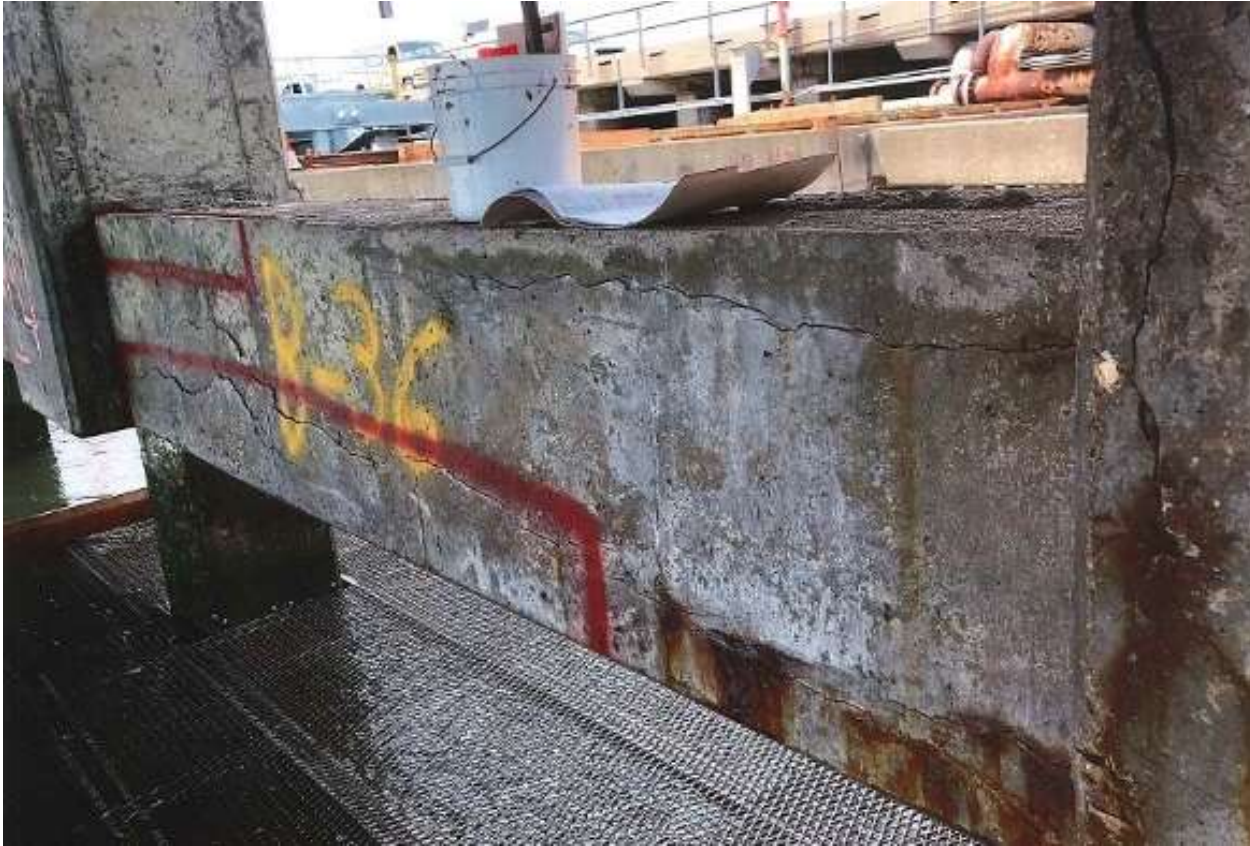
Concrete Beam with Cracks & Rust Stains
