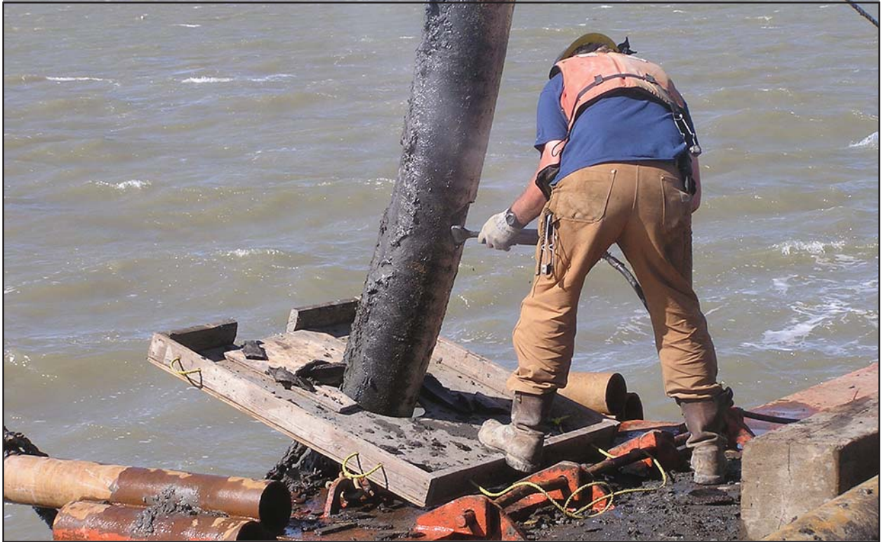
MARINE CREWMAN USING A PNEUMATIC CHISEL TO REMOVE A BAND OF COATING FROM A SUSPENDED SEGMENT OF RECOVERED PIPELINE IN PREPARATION FOR CUTTING THE PIPELINE. THE DERRICK BARGE CRANE IS HOLDING THE UPPER END OF THE PIPE. THE WOODEN TRAY IS TEMPORARILY FITTED AROUND THE PIPE TO CAPTURE THE PIPE WEIGHT COATING AS THE BAND OF COATING IS REMOVED.
