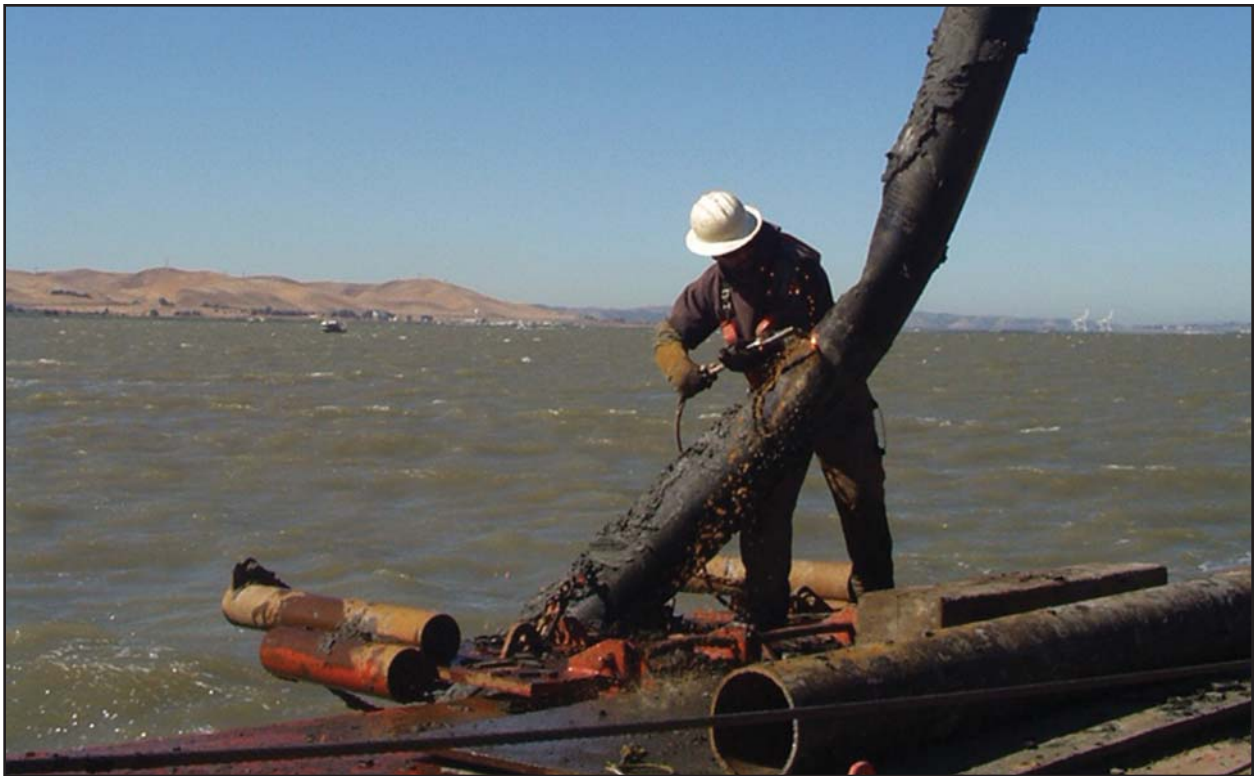
MARINE CREWMAN USING AN OXYGEN-ACETYLENE TORCH TO CUT A SUSPENDED SEGMENT OF PIPE. THE DERRICK BARGE CRANE IS HOLDING THE UPPER END OF THE PIPE AND WILL SWING THE CUT PIPE SEGMENT OVER TO AN ADJACENT MATERIALS BARGE ONCE THE CUT IS COMPLETED.
