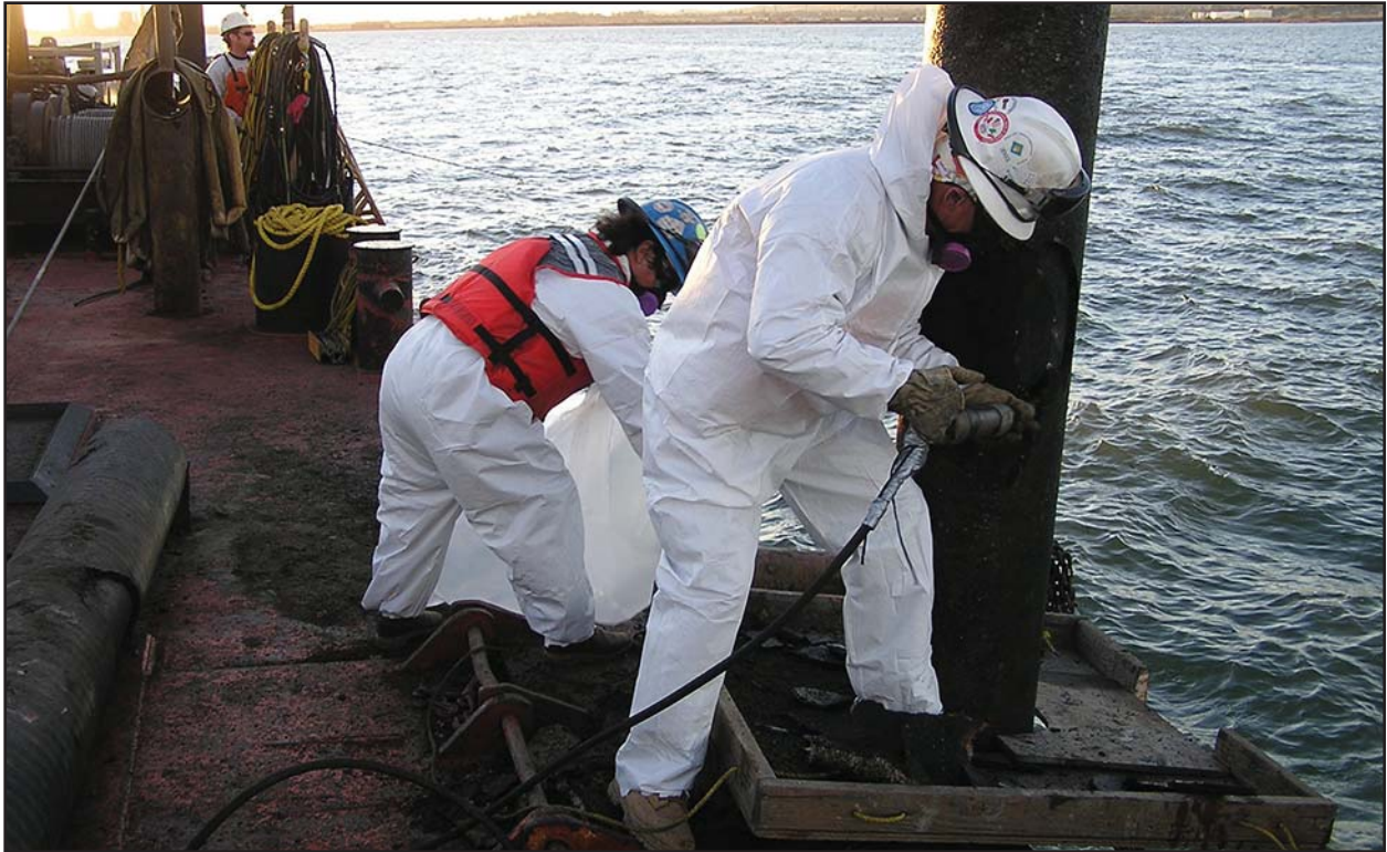
A CREWMAN CERTIFIED IN HANDLING ASBESTOS USES A PNEUMATIC CHISEL TO REMOVE A BAND OF COATING FROM A SUSPENDED SEGMENT OF RECOVERED PIPELINE IN PREPARATION FOR CUTTING THE PIPELINE. A SECOND CREWMAN RECOVERS THE PIPE COATING AND BAGS IT FOR OFFSITE DISPOSAL.
