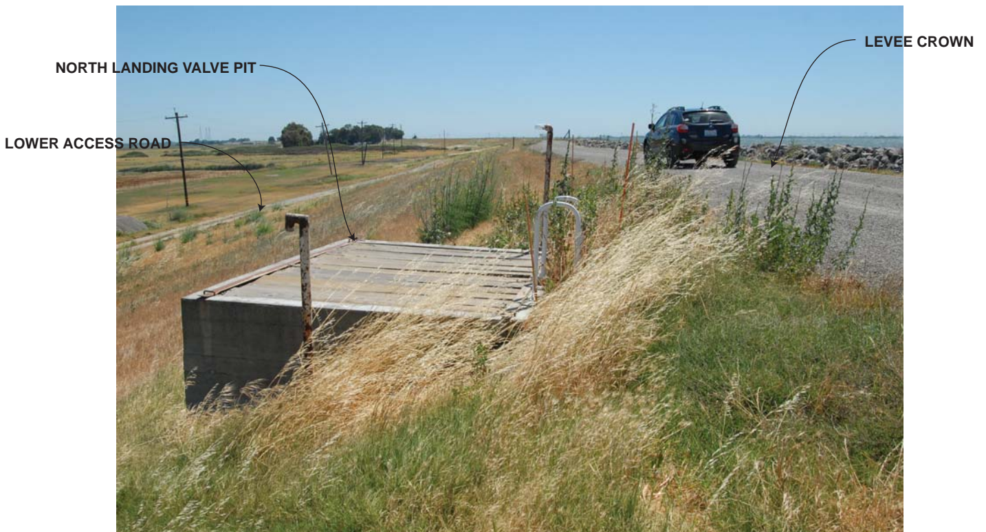
PHOTO 2 - VALVE PIT AT NORTH LANDING.
